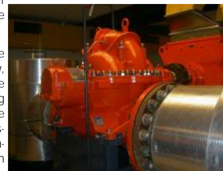
In July 2005 we completed the supply of Pumps for the heat distribution station, VEKS
